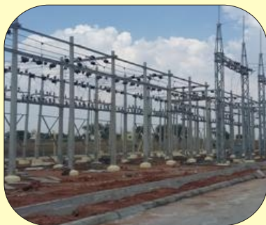
11kV DP Structure
