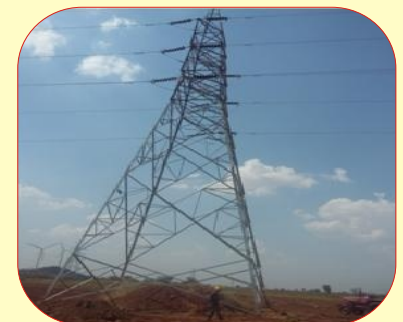
Transmission Line Tower
