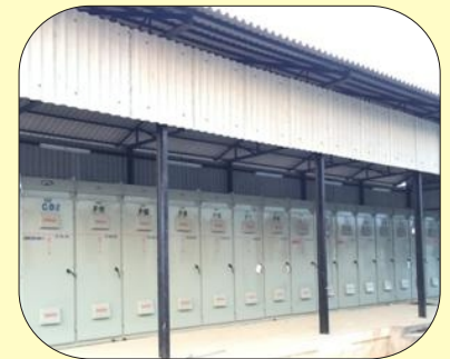
11 kV Switchgear room
