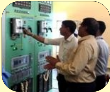
Charging 66/11kV SS
